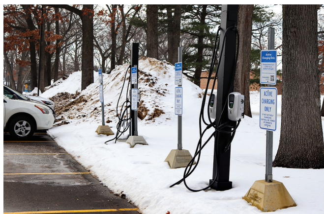
Charging stations installed in newly paved main parking lot.
